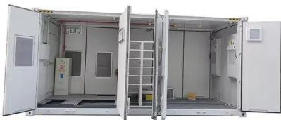
1075KW HH ESS
